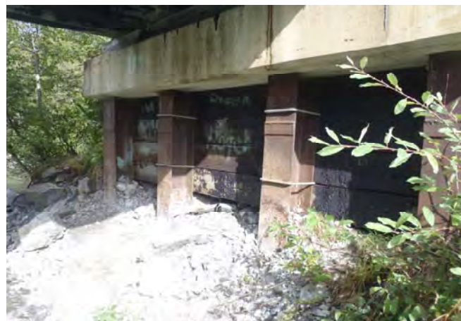
Figure 1-18: Likely end abutment, minor scour at toe of breast wall.
