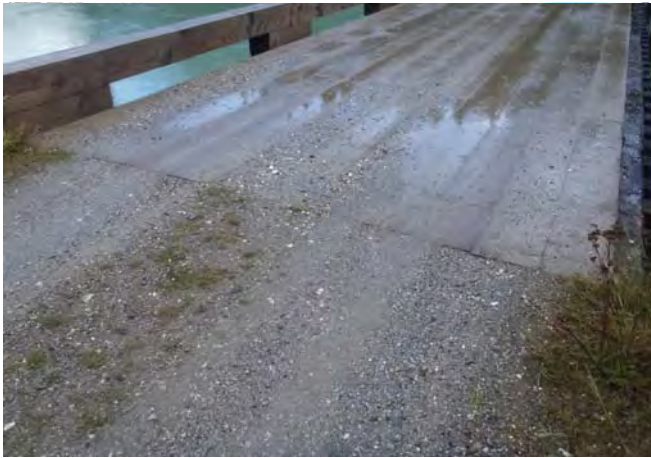
Figure 1-7: Likely end abutment deck end.
