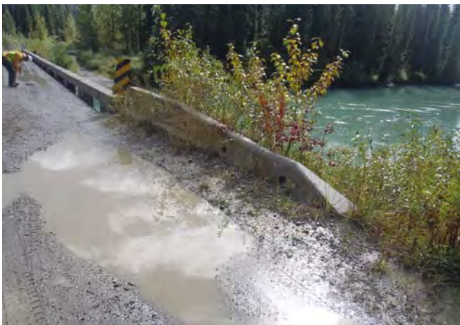
Figure 1-9: Typical misaligned barrier, wells end downstream shown.
