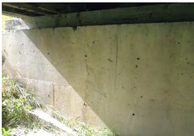
Figure 1-21: Wells end abutment, breast wall crack.
