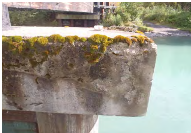
Figure 1-24: Pier cap downstream corner, minor spall and moss growth.
