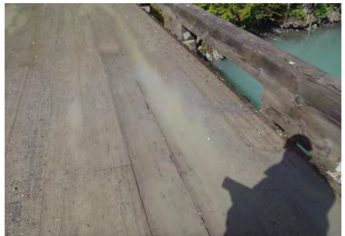
Figure 1-10: Typical curb rail condition, note ponding water.
