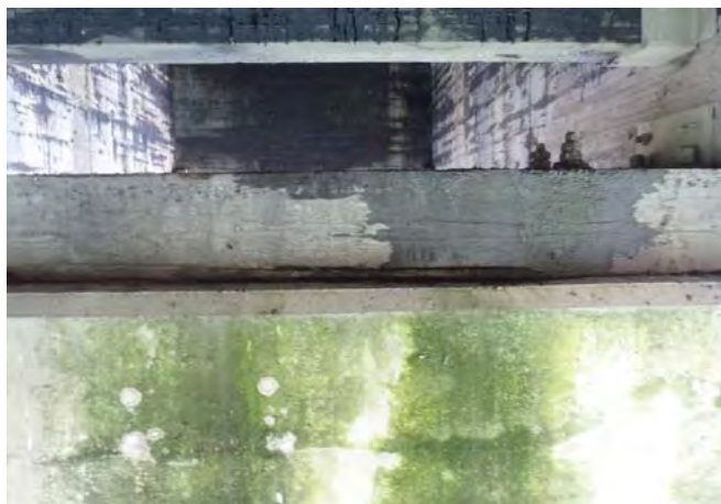
Figure 1-23: Pier sill, minor damage and moisture noted.
