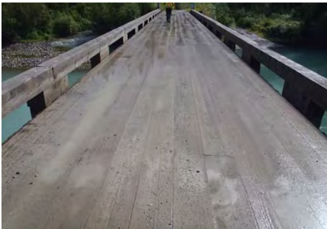
Figure 1-11: Typical deck condition.
